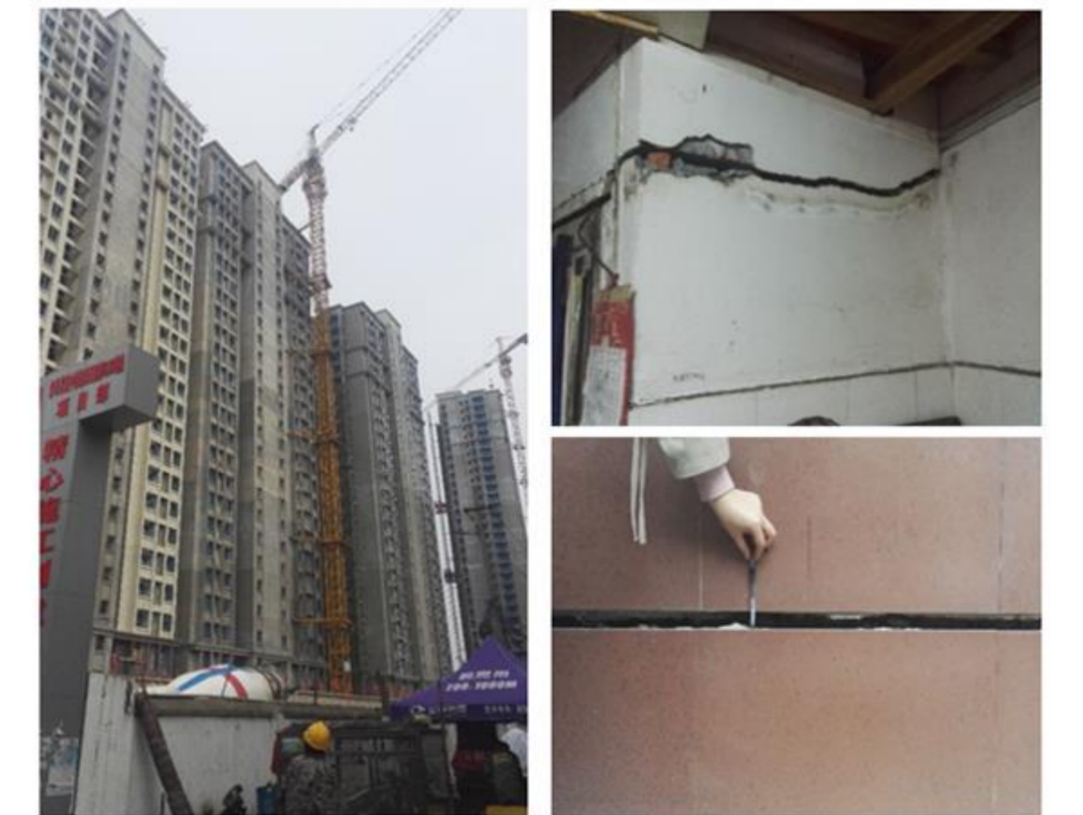
Figure4. Wall cracking in Changmatou built-up areas
